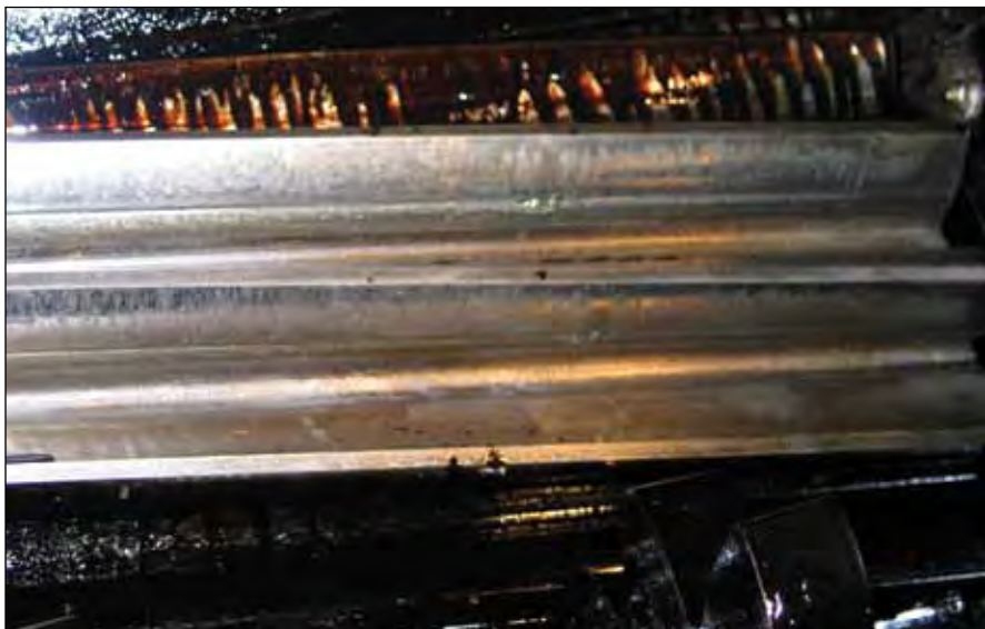
A kiln gear set showing distress due to insufficient viscosity (courtesy Rexnord Gear Group/Rexnord Industries LLC).
