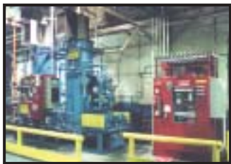
RX® Gas Generator and Controls
