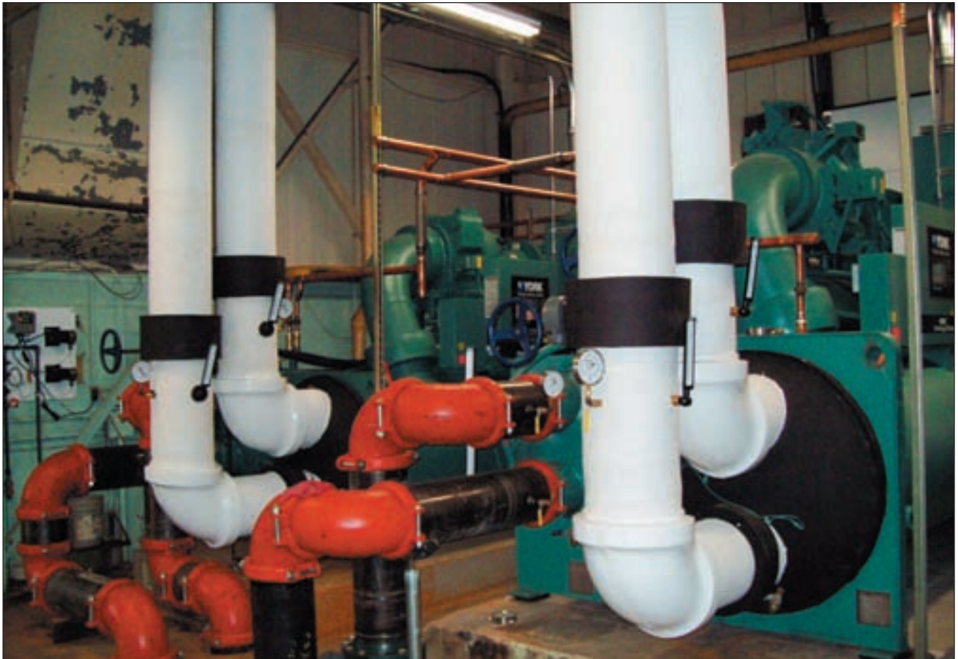
Gleason Cutting Tools installed a centralized chiling system to conserve energy and reduce shop floor costs (Courtesy of Gleason).
