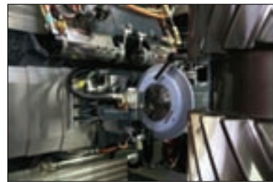
Workers (above) prepare the excavation prior to installation. Sixty yards of steel-reinforced concrete were poured to accommodate the machine's base. Another 16 yards of concrete were used around the machine's base in support of the housing. The machine is capable of producing gears with AGMA class 14-15 accuracies.
