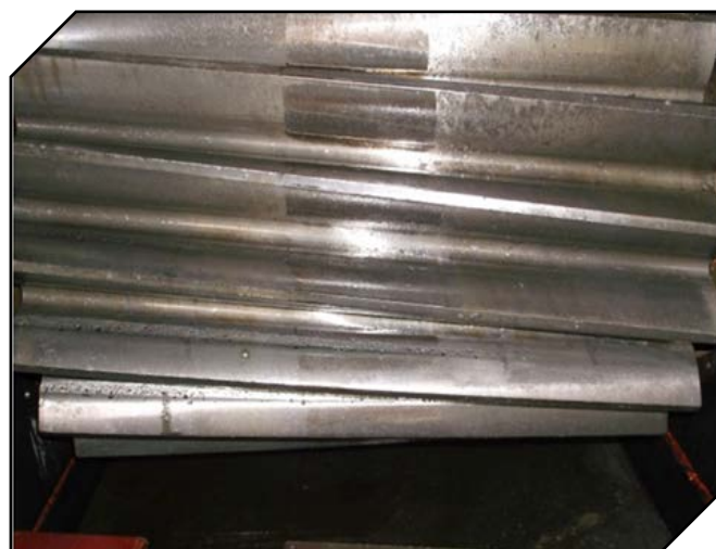
Figure 1 Example of girth gear misalignment: girth gear driving pinion end is aligned to the reducer, causing misalignment between the girth gear teeth and driving pinion teeth (courtesy HMC).
