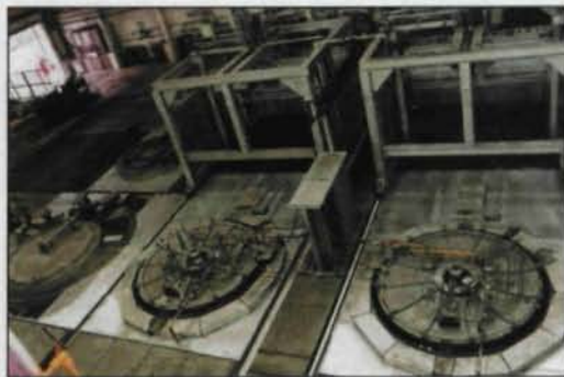
Figure 2—New gas-carburizing furnaces. Maximum measurements of a gear can be 2.5 m in diameter, 2.5 m in height, and 15,000 kg in weight. Carrier gas is a mixture of methanol and nitrogen, enriching gas is propane.
