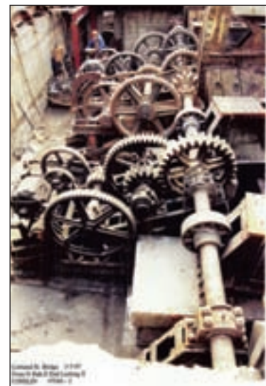
A look at the gear set that powers the Cortland Street Bridge. (Photo courtesy City of Chicago.)
