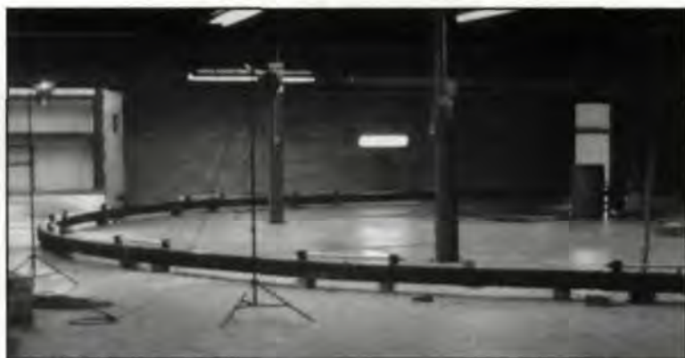
Fig. 2 — A view of the floor as the gear was being assembled gives some idea of the magnitude of the gear. A special site had to be found for the assembly process, and every piece fit together and leveled properly.
