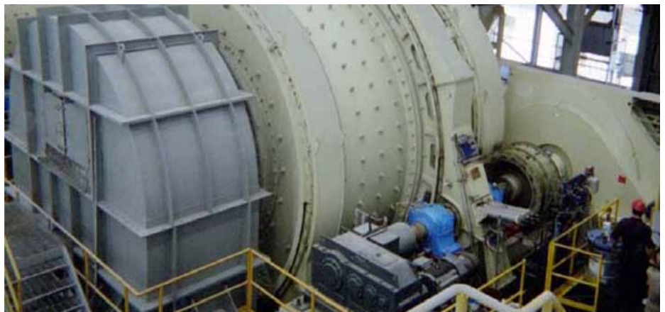
Figure 1 Grinding mill installation.
