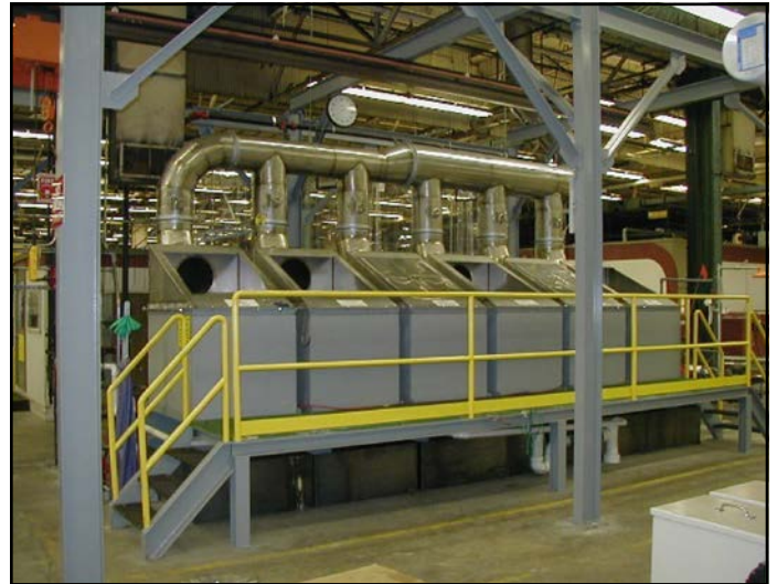
Figure 1 Series of tanks for acid etching in a gear manufacturing facility.
