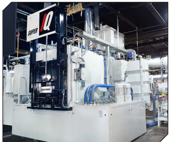
Figure 4 Clean integral quench carburizing furnace with no toxic gases and precision, high-volume carburizing for gears, shafts, and various other components.
