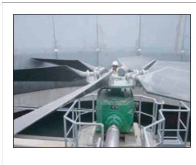
Figure 3—Installed air-cooled fan.
