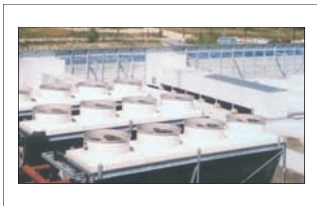
Figure 1—Air-cooled condenser bank.
