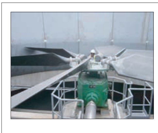
Figure 3—Installed air-cooled fan.
