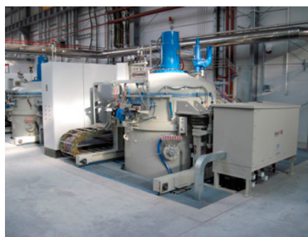
The new SECO/Vacuum Pit-LPC vacuum furnace.
