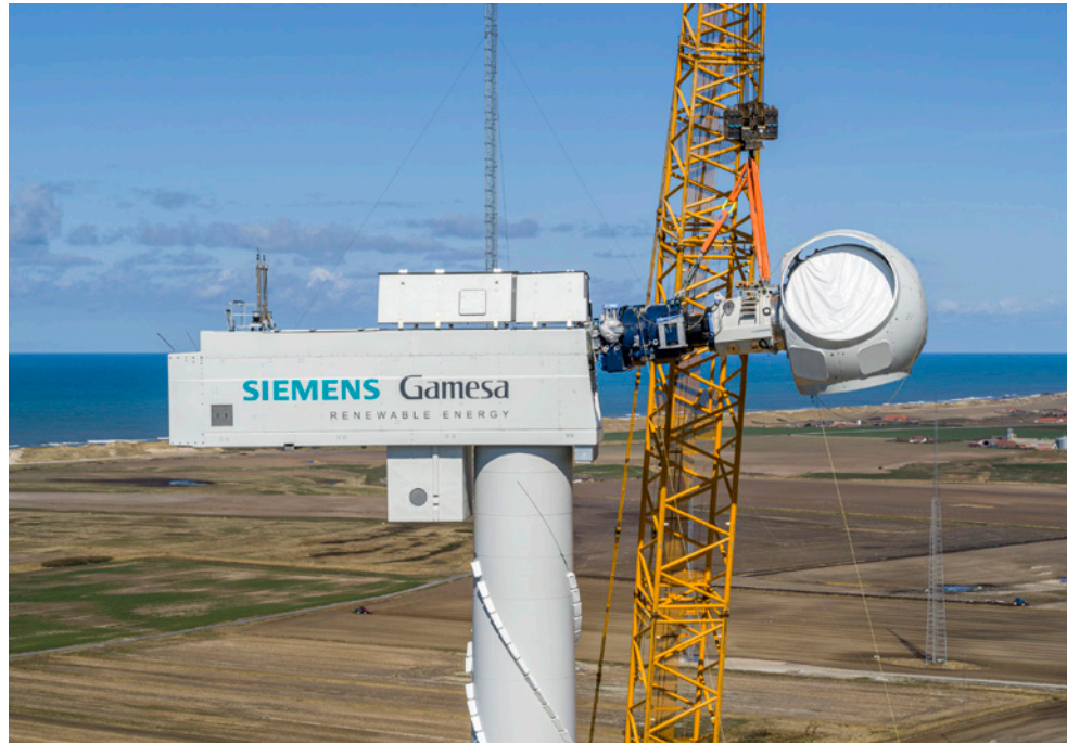
Figure 1—Drivetrain assembly of SGRE 5X 170 prototype turbine in Hovsøre wind farm (Denmark).
