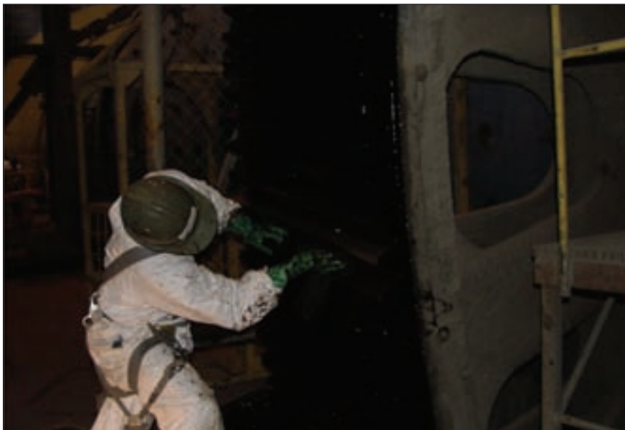
Drago examines a SAG mill gear, which is about 35 feet in diameter, at a copper mine in Chile in order to determine the cause of tooth surface fatigue damage.
