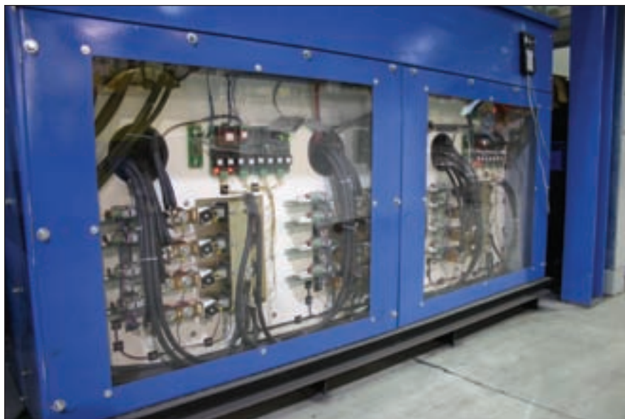
Solar Atmospheres boasts an energy efficient dry power supply.
