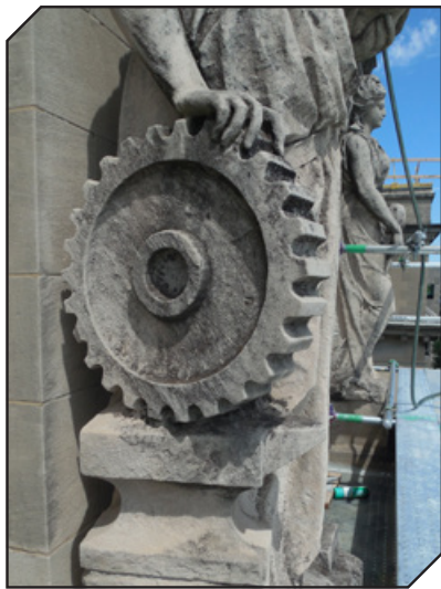
Part of a statue, this stone gear was damaged by acid erosion, creating a more porous surface on which black grime accumulated.
